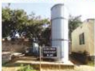
Waste Water Treatment Plant
